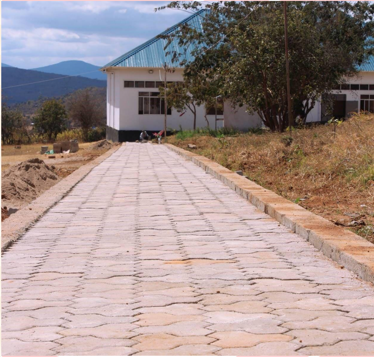
The 750M2 paving project at Sunflower Pre and Primary School began and was finished
